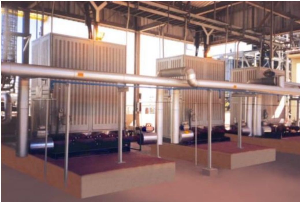
Figure 12 -Typical assembled Difhemi of 900 kw each one
