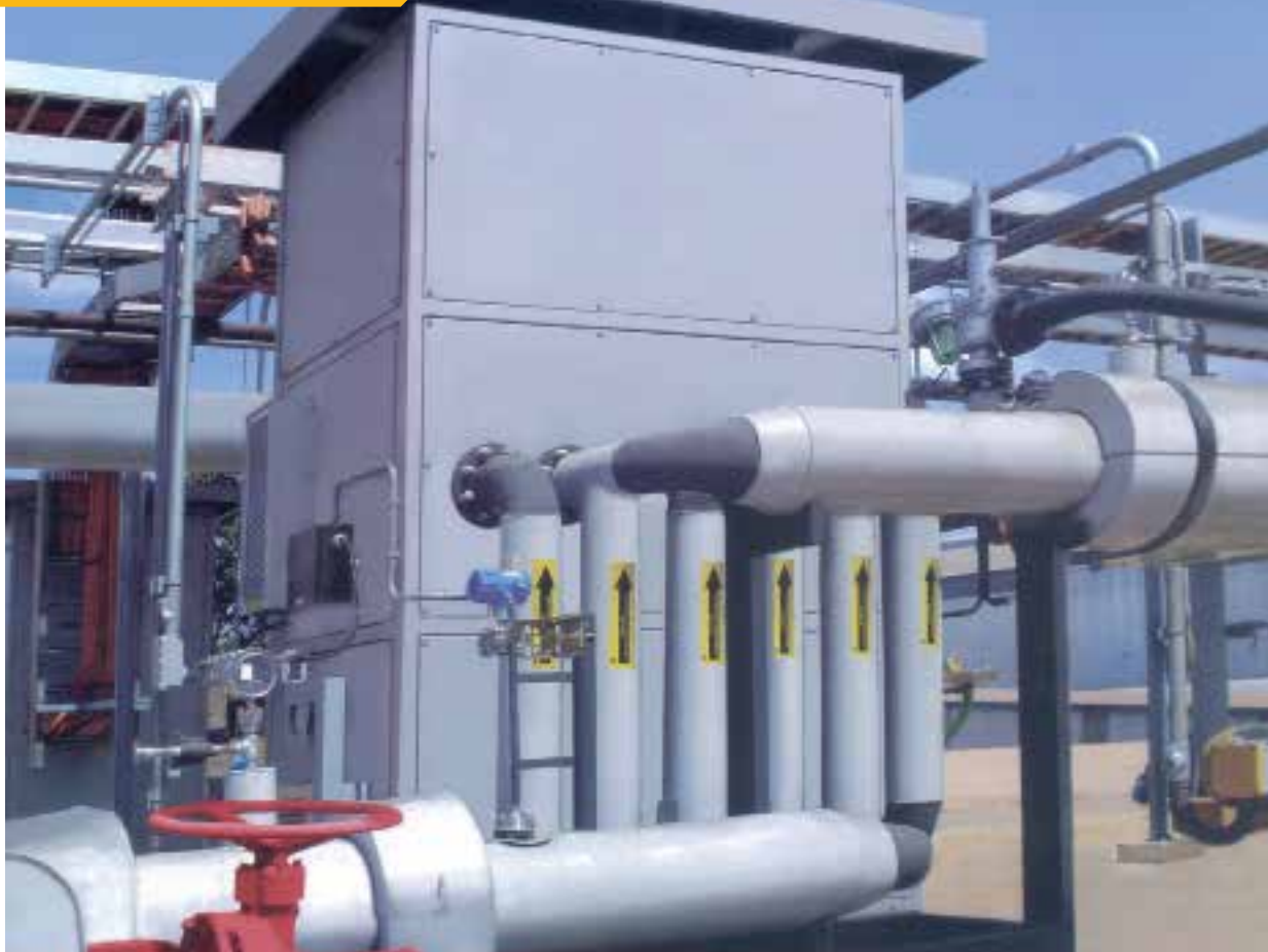
A DIFHEMI system in situ
